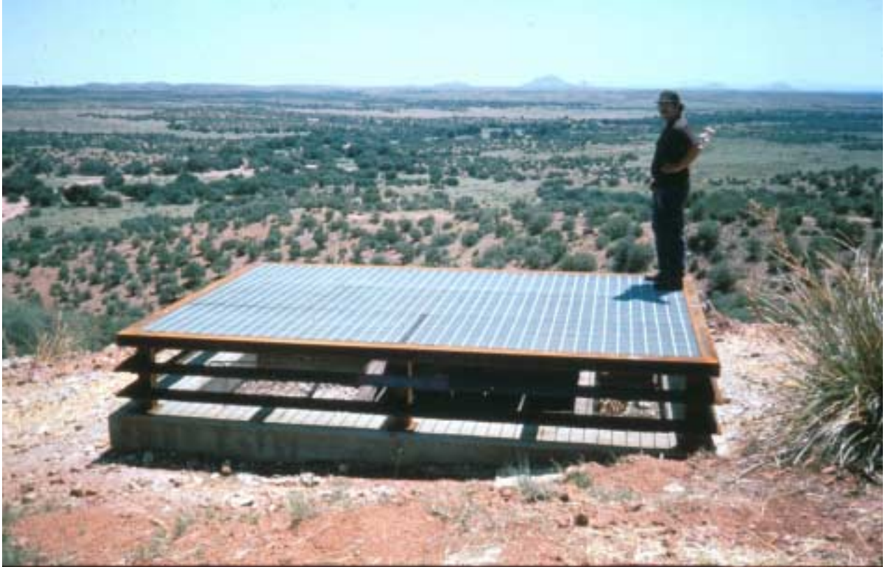
Angle-iron cage constructed over a shaft in New Mexico. This type of structure is suitable for entrances that must be kept open to maintain airflow but are not used by bats. (Photograph credit, John Kretzmann, New Mexico Mining and Minerals Division, Sante Fe, New Mexico).
