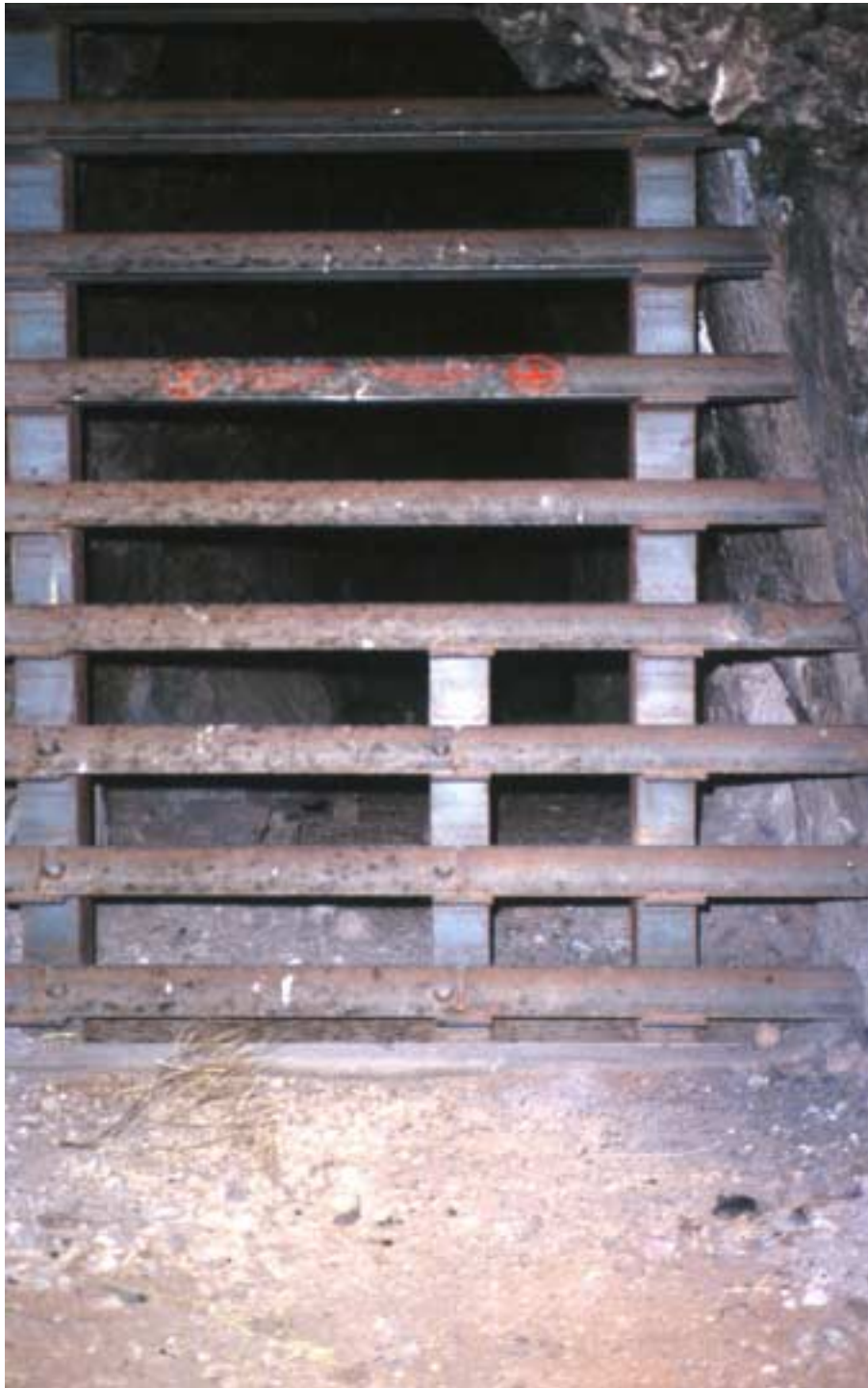
Angle-iron gate in New Mexico designed by John Kretzmann. The left side of the bottom three bars are attached with McGard security bolts. These bolts require a uniquely patterned socket for installation and removal and have proven a very effective means of securing removable bars. (Photograph credit Robert R. Currie, U.S. Fish and Wildlife Service, Asheville, North Carolina.)
