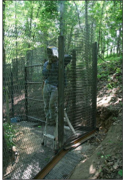
Left: Roy Powers measuring for the removable bar at the Basic Gate section of the Powers Fence. Right: Welder Jerry Fant fills in the top gaps above the columns. Both photos at Bellamy Cave, by Jim Kennedy.
