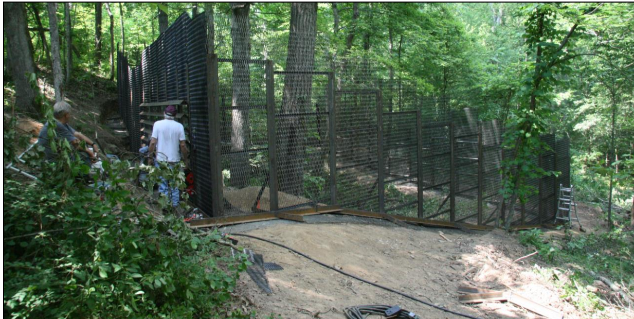
Powers Fence being constructed around Bellamy Cave, Montgomery County, Tennessee. The late Mastergater Roy Powers is in the front left of the photo, in white T-shirt. Photo by Jim Kennedy.
